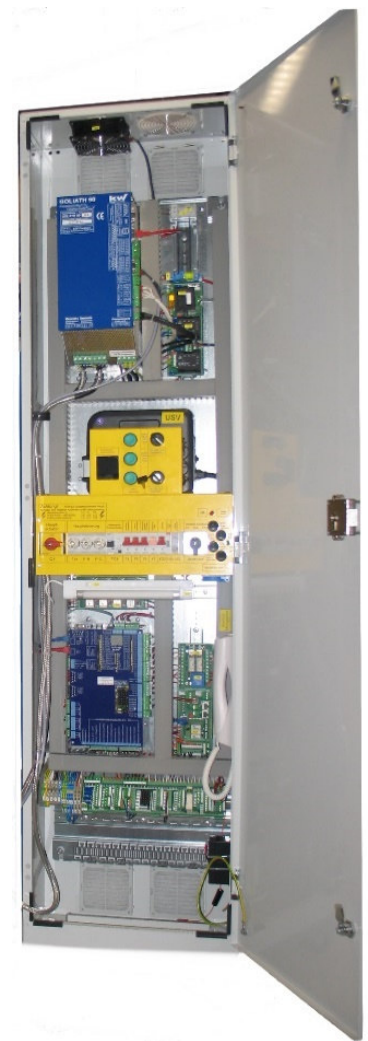
Cabinet KW03Z with internal Inverter
