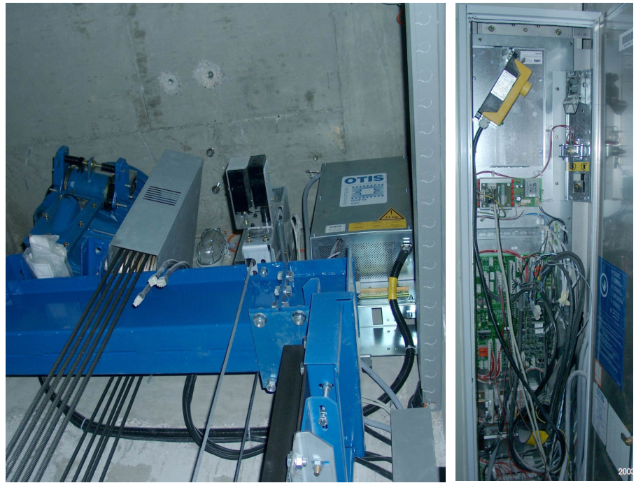
Original equipment –Motor & Inverter shaft-head
