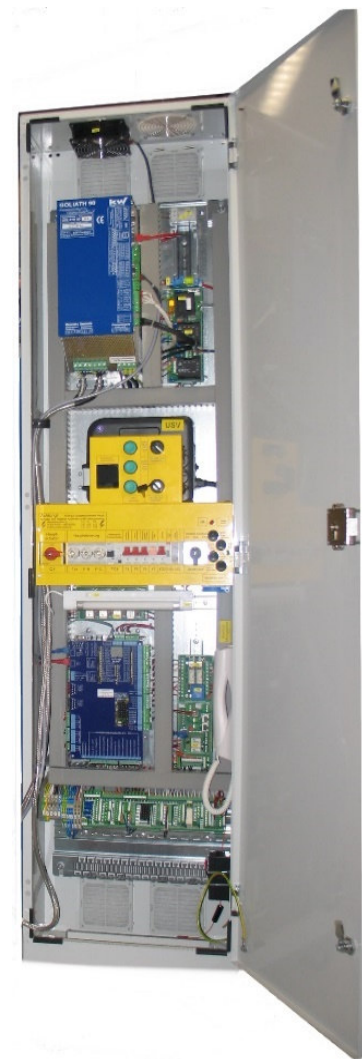
Cabinet KW03Z with internal Inverter
